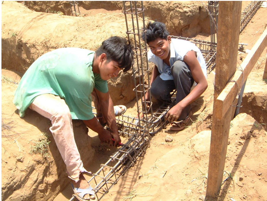
Young people involved in constructing a community centre in León South East
